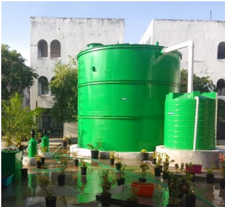
1 Tonne capacity Biogas Plant converts Food Waste generated in the Institution Mess to Biogas replacing 3 commercial cylinders daily
