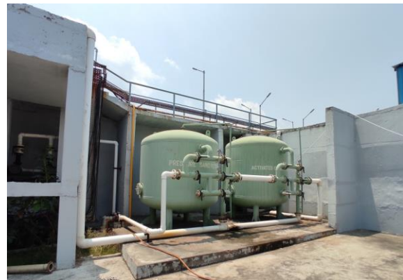
Figure 9: Water treatment unit
