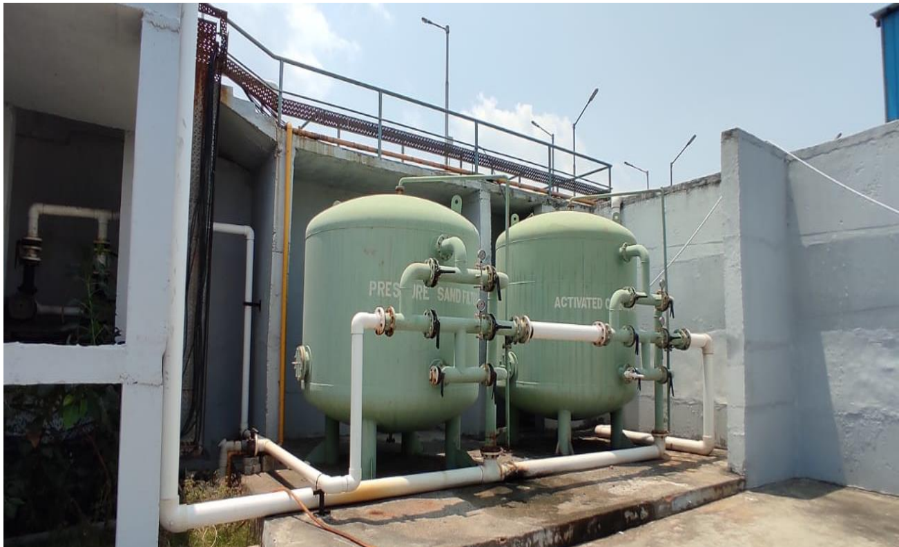
Figure 33: STP-Sand Filtration, Carbon Filtration
