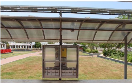
Figure 41: Solar Panels with Controller
