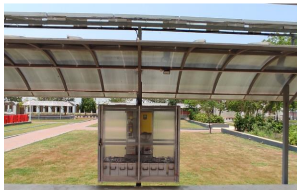
Figure 15: Solar Panels with Controller
