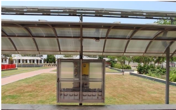
Figure 23 Solar panels with controller
