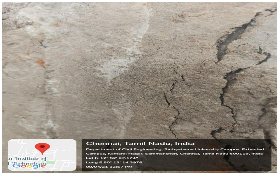
Fig 5.4 cracks on the sides of CFRP fully wrapped beam
