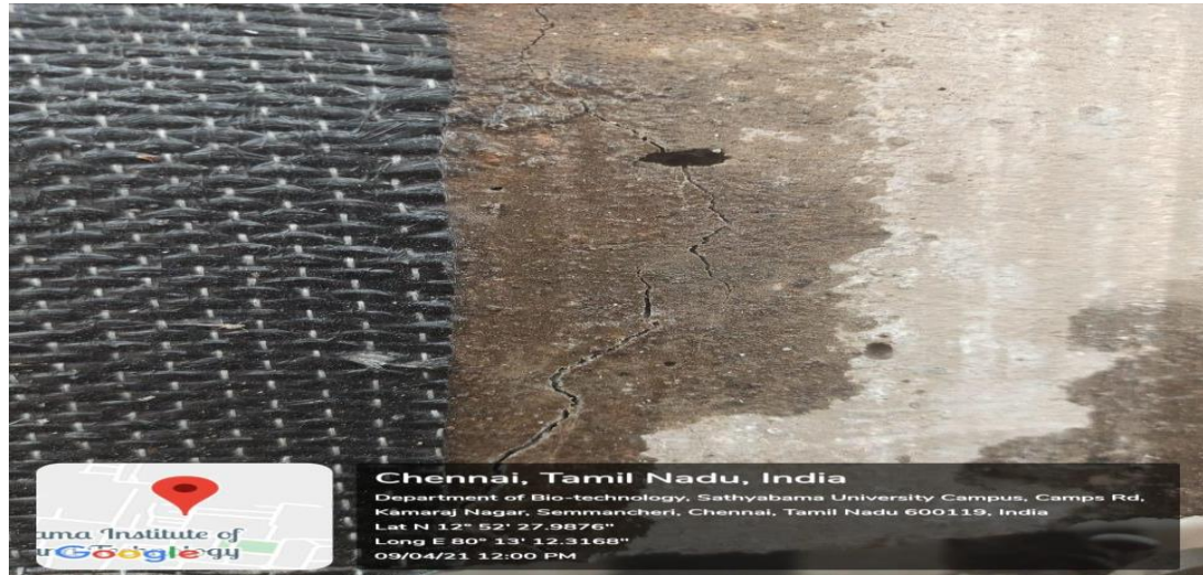
Fig 5.8 First crack on CFRP wrapped beam with 100 mm interval
