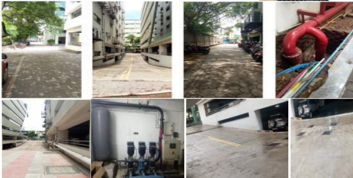
Fig 6.6 View of chiller plant and Air handling unit
