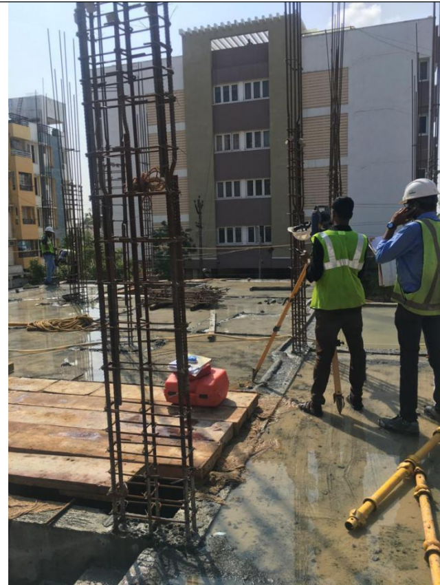
Column Starter dimension checking(B-2)
