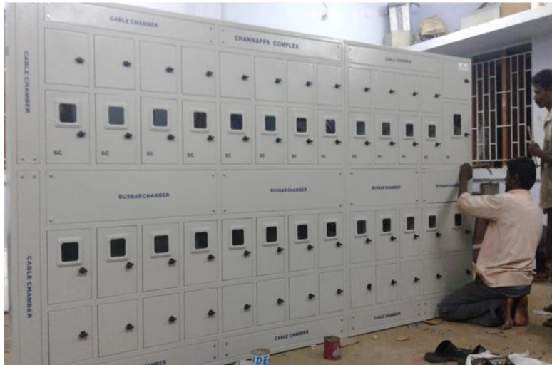
Fig 6.2 Panel Boards with 24-meter boxes
