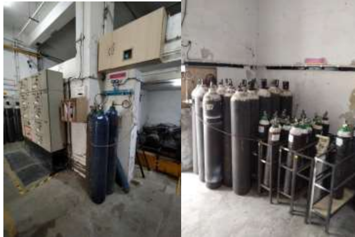
Fig 2.25 Kauvery Hospital Portable Cylinders
