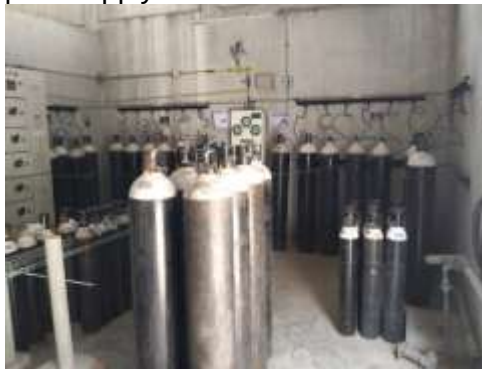
Fig 3.10 Kamakshi Memorial Hospital Oxygen manifold
