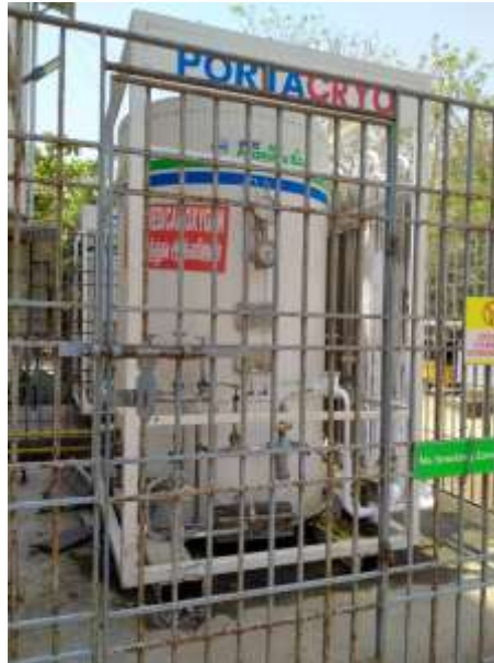
Fig 3.9 Kamakshi Memorial Hospital Liquid oxygen
