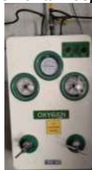
Fig 3.11 Kamakshi Memorial Hospital Oxygen Control Panel
