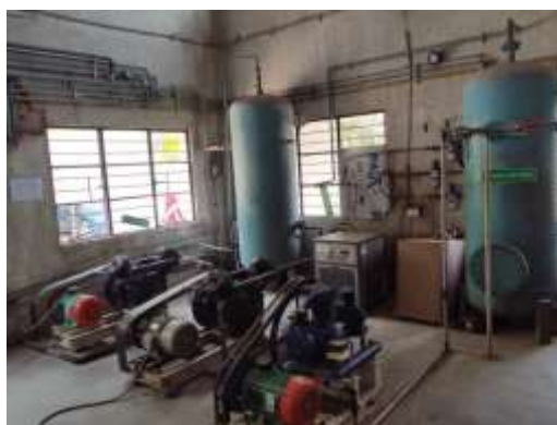
Fig 3.13 Kamakshi Memorial Hospital Air and Vacuum Compressor
