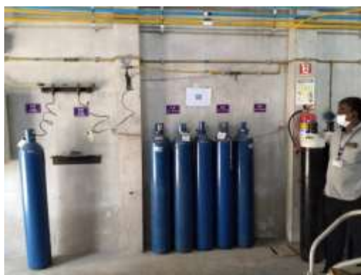
Fig 3.12 Kamakshi Memorial Hospital Nitrous Oxide manifold
