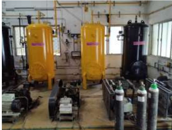
Fig 2.22 Kauvery Hospital Air and Vacuum Cylinders
