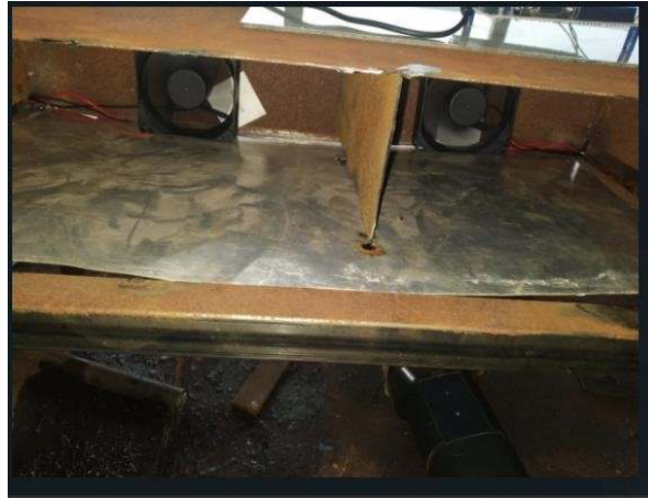
Fig 4.14 Fabrication Fans fitted on either side of the cooling and heating box.
