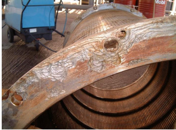
Fig. No. 2. Electro chemical corrosion
