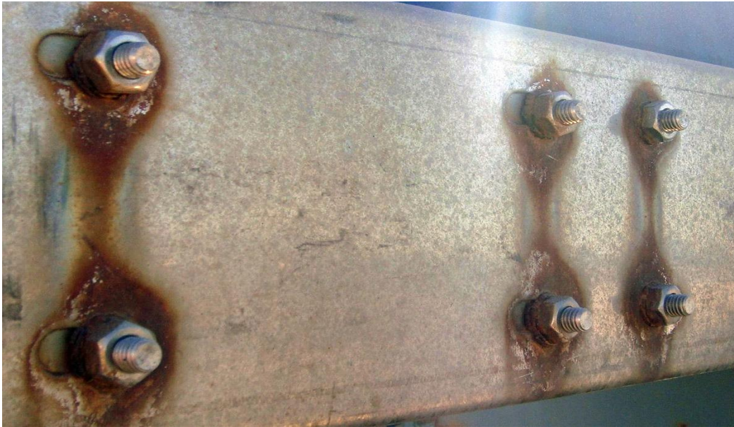
Fig. No. 8. Galvanic Corrosion
