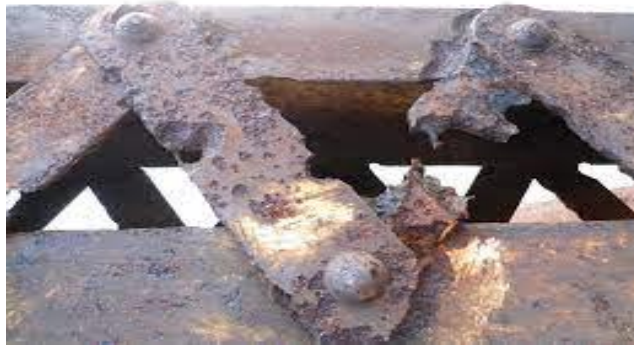
Fig. No. 4. Pitting Corrosion
