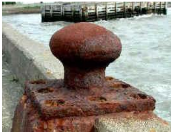
Fig. No. 3. Uniform Corrosion
