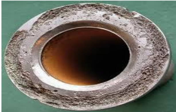
Fig. No. 5. Crevice Corrosion
