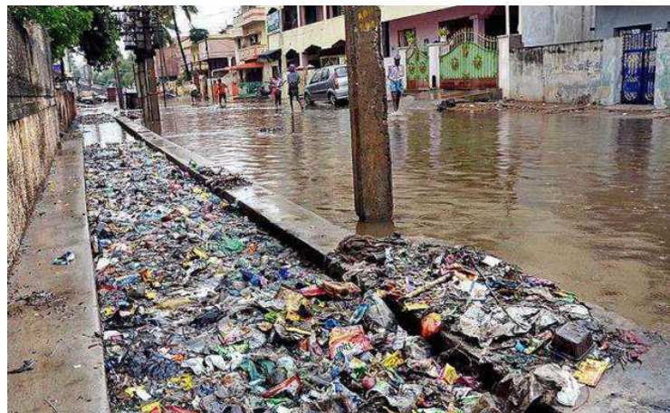
Fig1.2:Deposition of solid waste in drainage scrap
