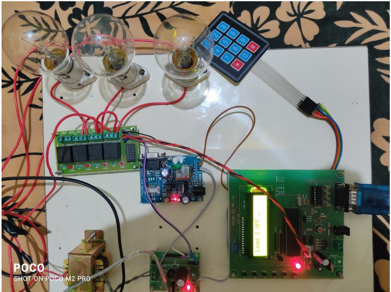
Fig. 4.27 Status of the Load 3 in OFF Position
