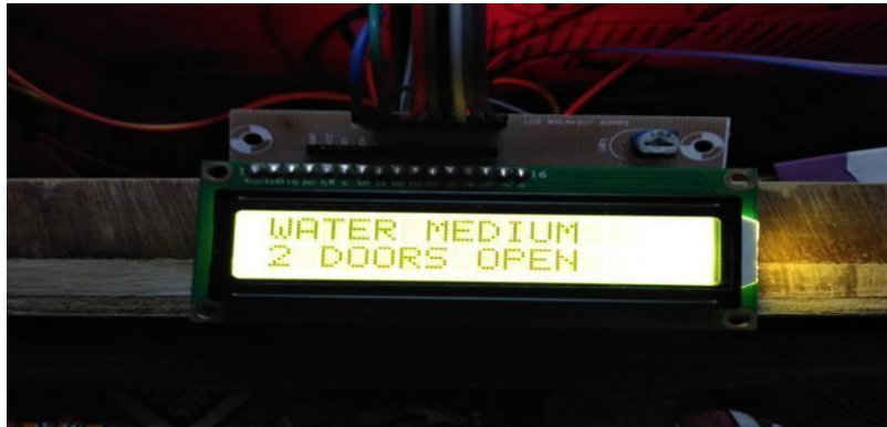
Fig 5.3 Water Level – MEDIUM
