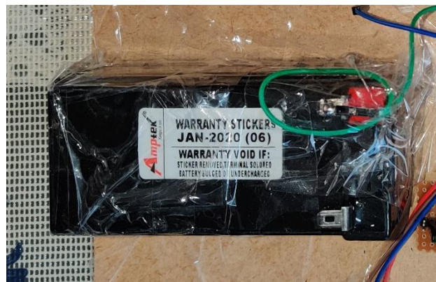
Fig: 4.23: Power Supply Battery
