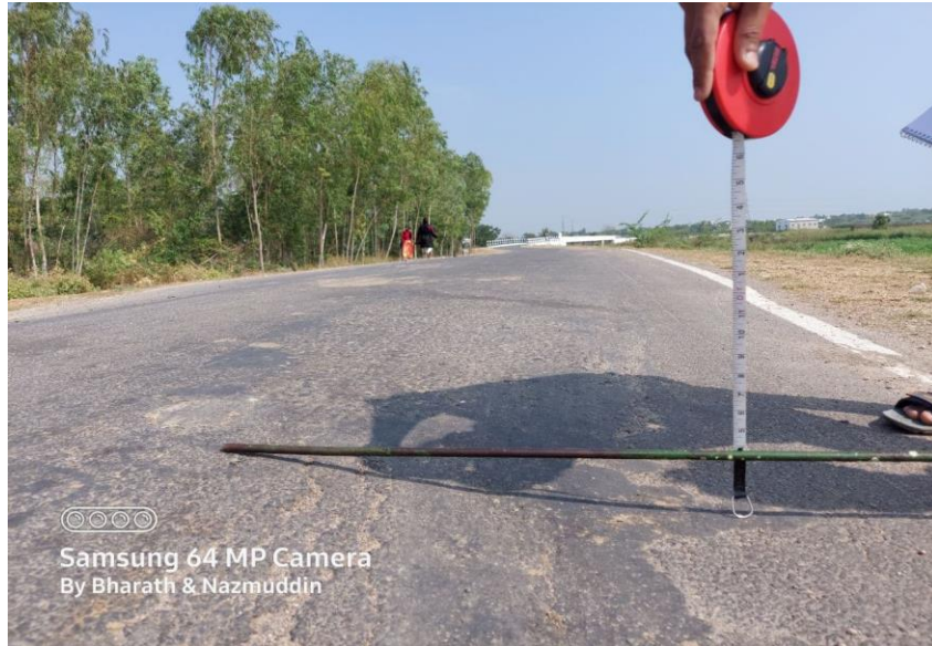
Fig: 3.4: Shallow depression at chainage @ 0.581- 0.595 KMS
