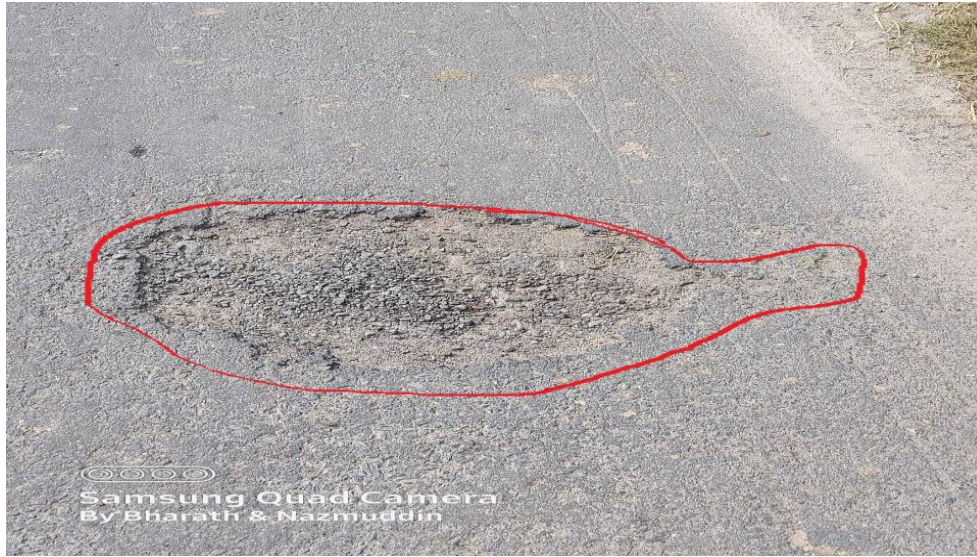
Fig: 3.2: Pothole at chainage @1.495 KMS
