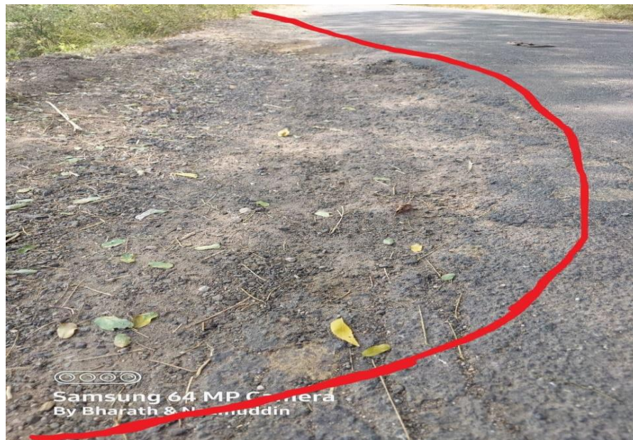
Fig: 3.5: Edge cracking at chainage @ 1.682 KMS
