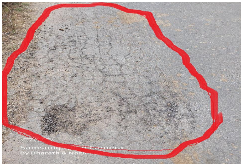
Fig: 3.3: Alligator cracking at chainage @1.092 KMS
