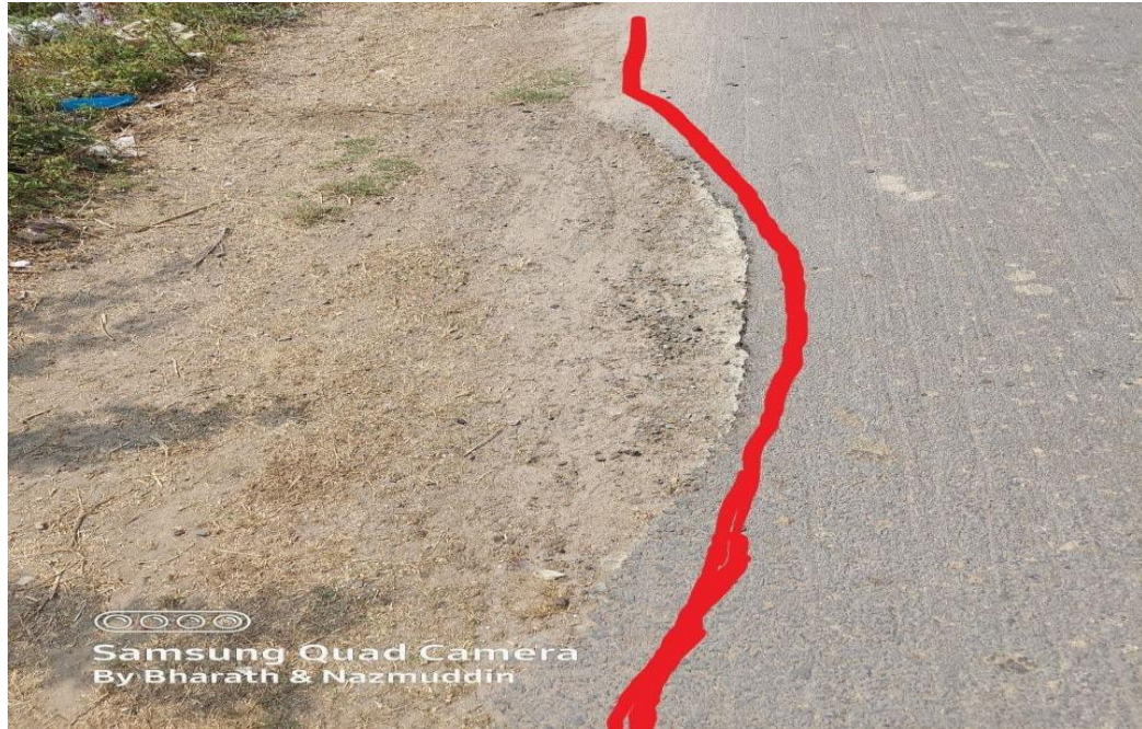
Fig: 3.6: Edge breaking at chainage @ 0.095 KMS
