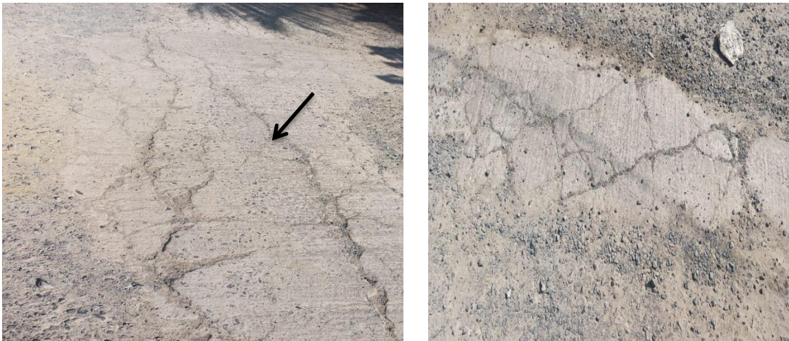
Fig:4.2 :Scaling of Cement Concrete.
