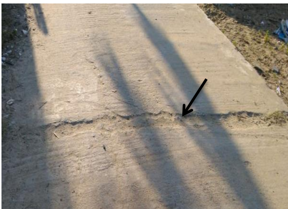
Fig:4.3 :Joint Spalling in Rigid Pavement.
