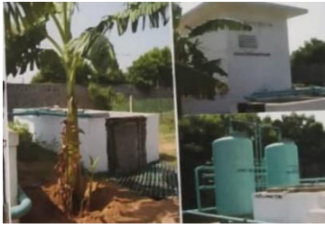
Figure 2. 28 Sewage treatment plant
