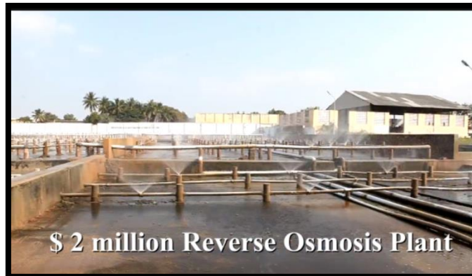
Fig.1.83. Figure shows RO Plant of KH Exports
