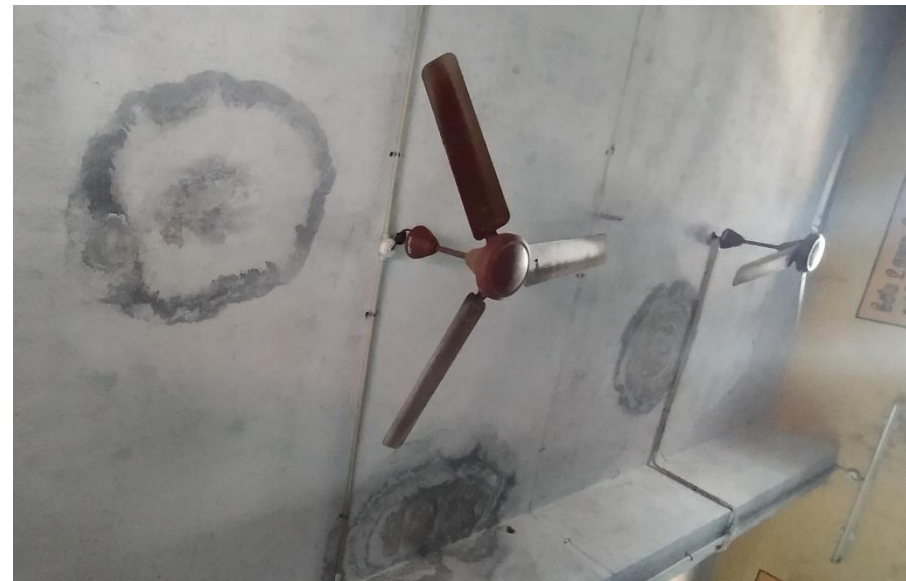
Leaking of celing
