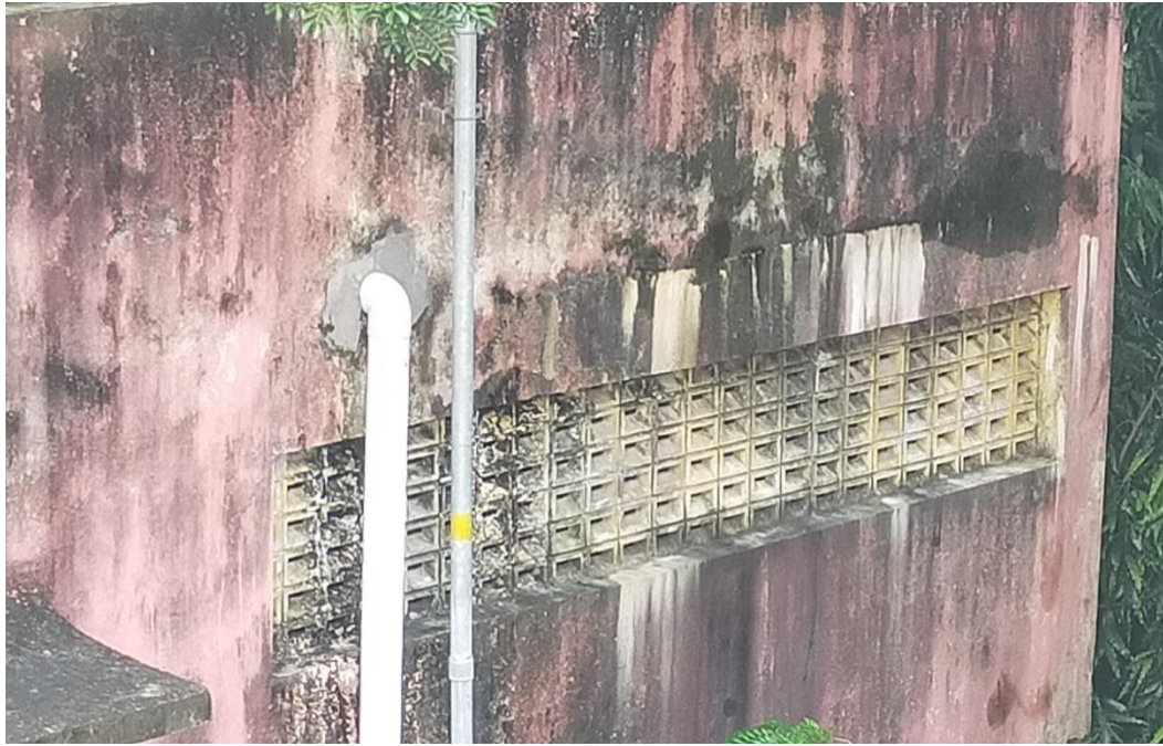
Exterior of the block with cracks
