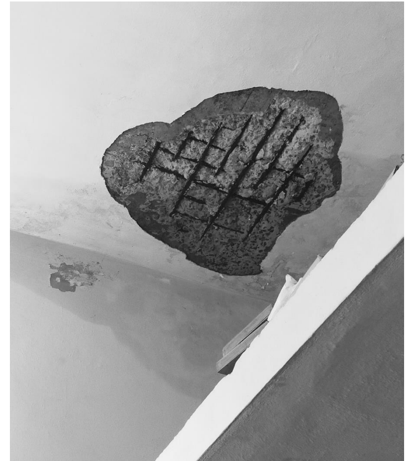
Cracks in ceiling
