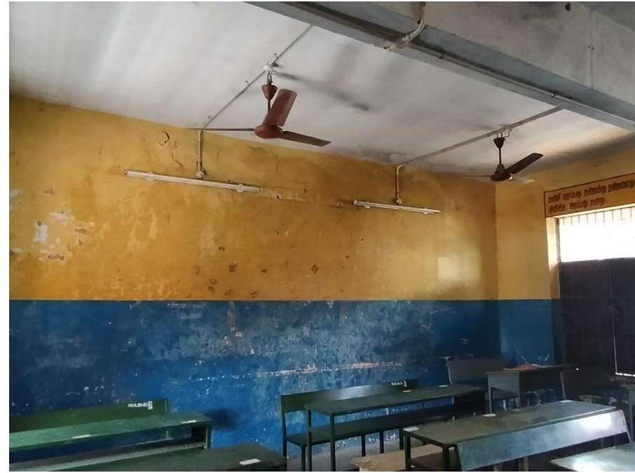
Leaking of walls
