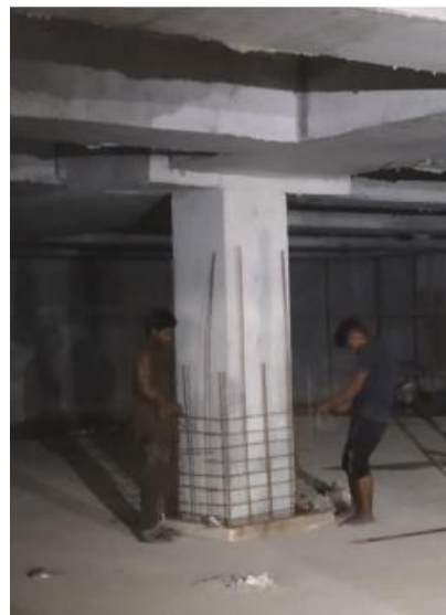
Hacking of column
