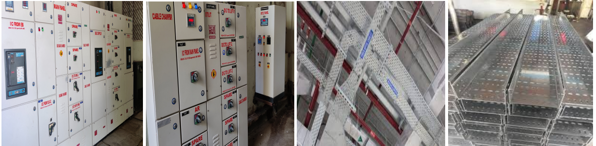
Fig 3.4 panel boards , bus ducts
