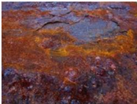
Fig. 1.4: Images of Cor-ten A588 steel when exposed to chloride (source https://distressedmetals.com/corten/limitations/ )
