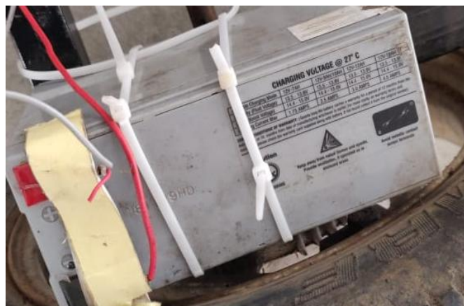
Fig 4.10: Lead acid Battery
