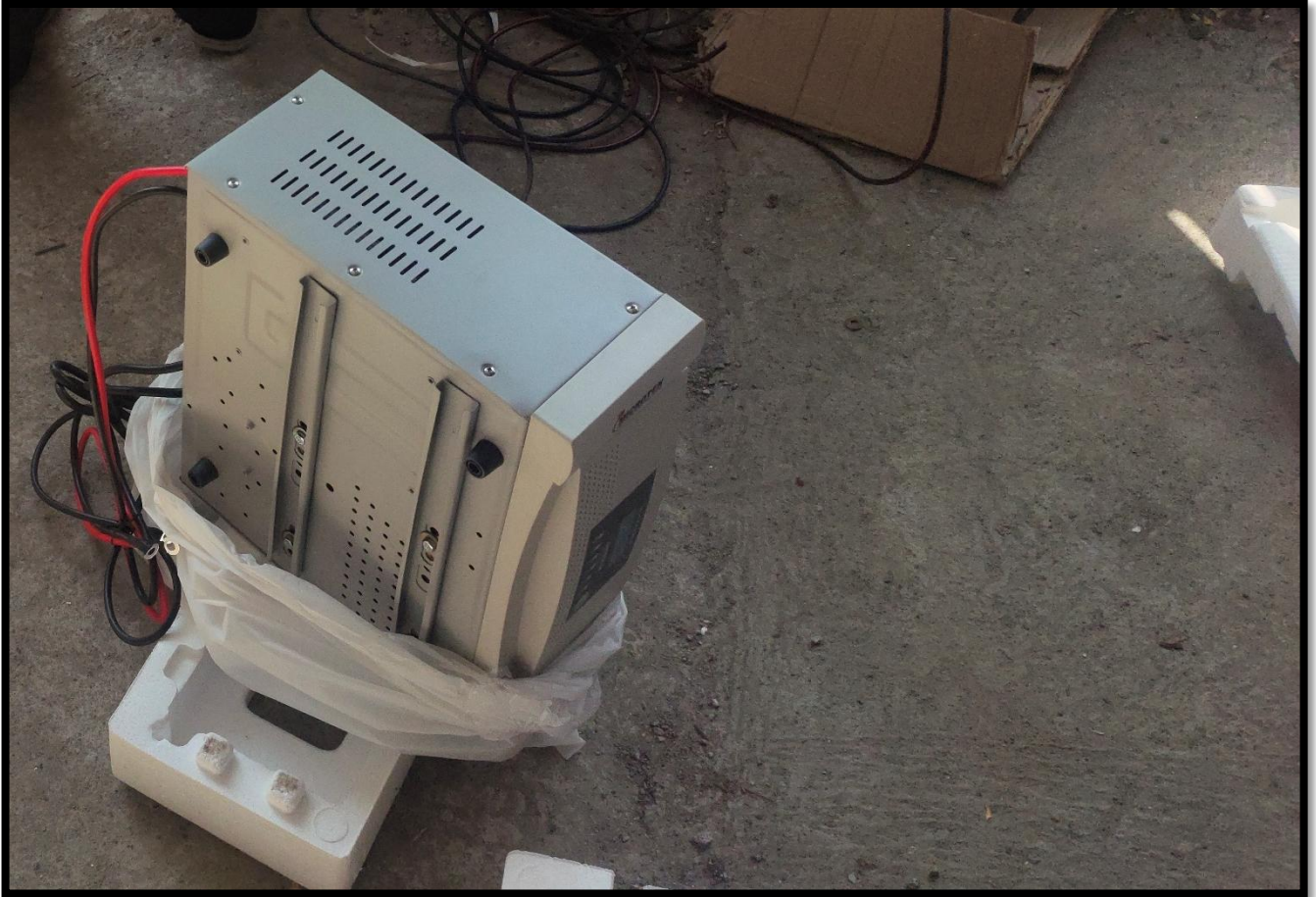
Fig 4.4: Inverter with inbuilt charge controller.
