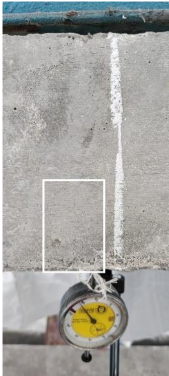
Fig:5.3 Creack of beam
