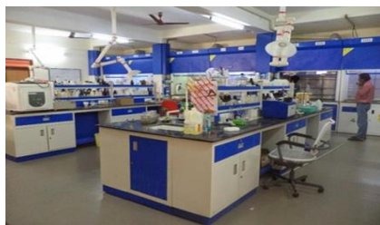
Fig 1: Modular lab, Fume hood & Spot Extraction System
