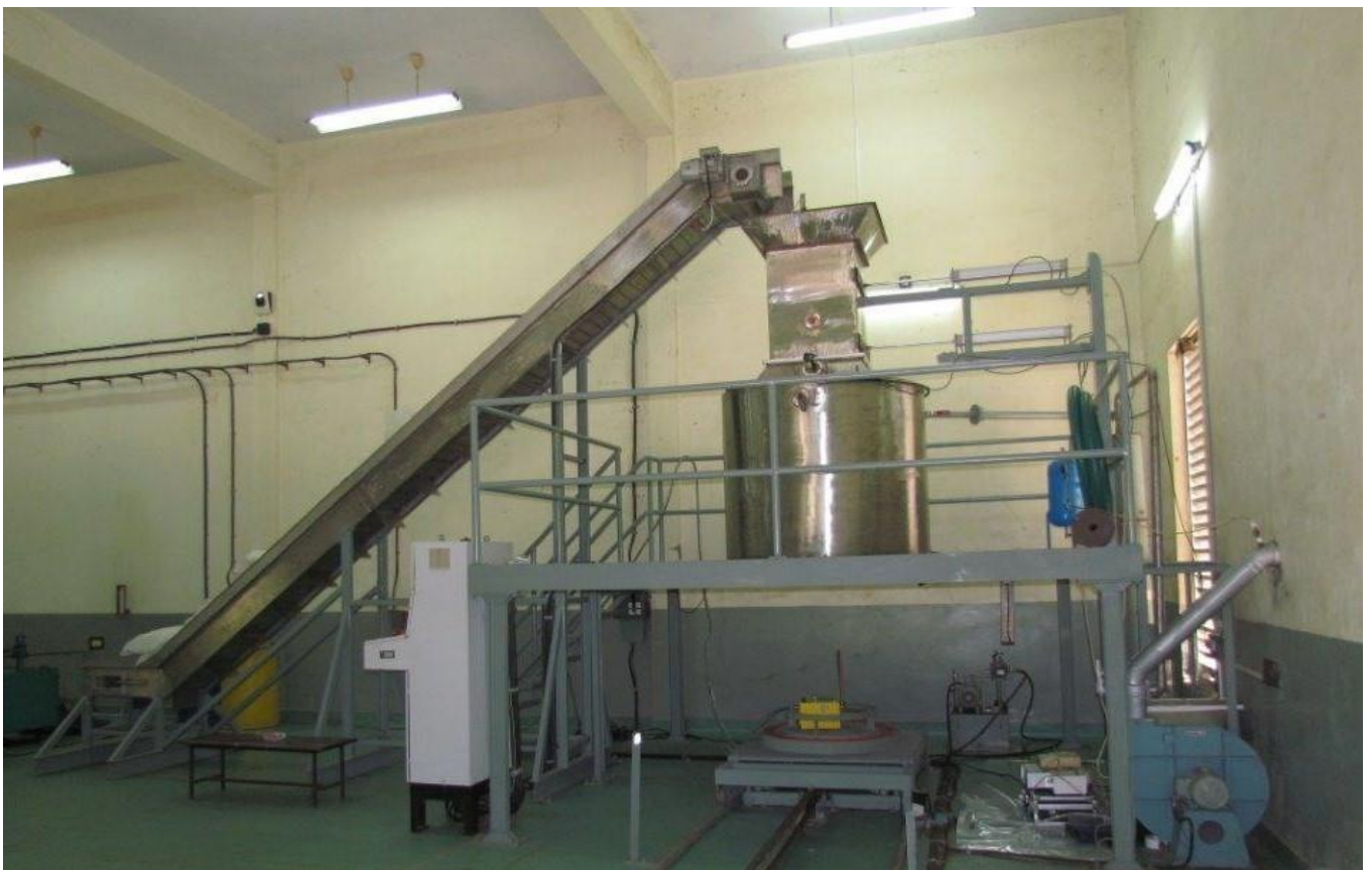
Fig: 2.4: Melt densification Unit
