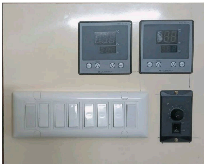
Figure 4.14: Power Supply Board
