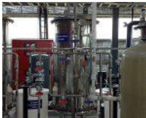
DM Plant 6000 LPH
