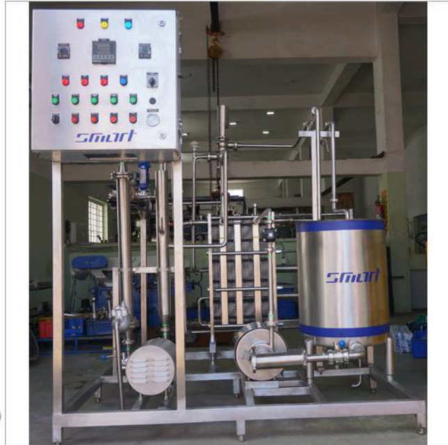
UHT PLANT IN AAVIN
