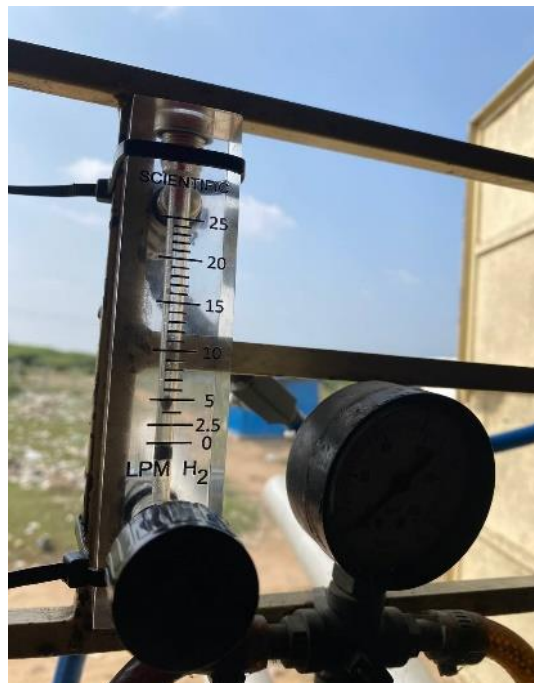
Fig. 4.3 Flow Regulator of Hydrogen gas
