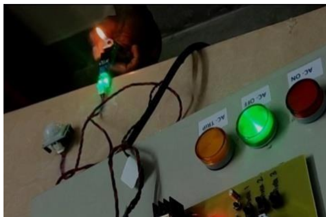
Fig. 11. Demonstration of activation of Fire sensor by naked flame.
