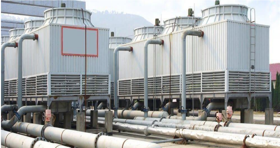
Figure 1.2: Depicts the typical installation of cooling tower in a central air-conditioning plant
