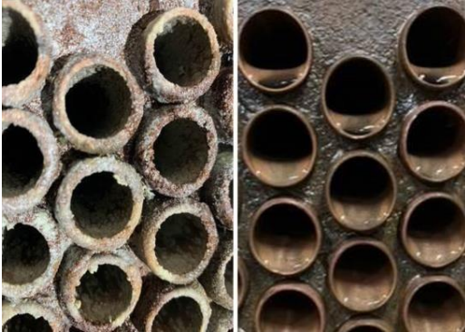
Figure 1.5: Shows condenser tubes before and after de-scaling
