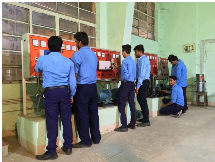
Figure 1.3 NSIC Electrical Room
