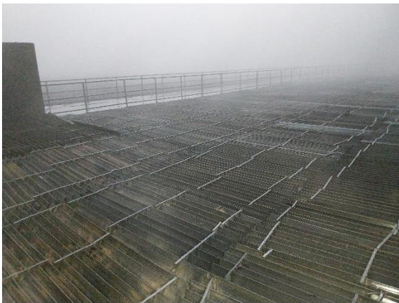
Inside cooling tower
