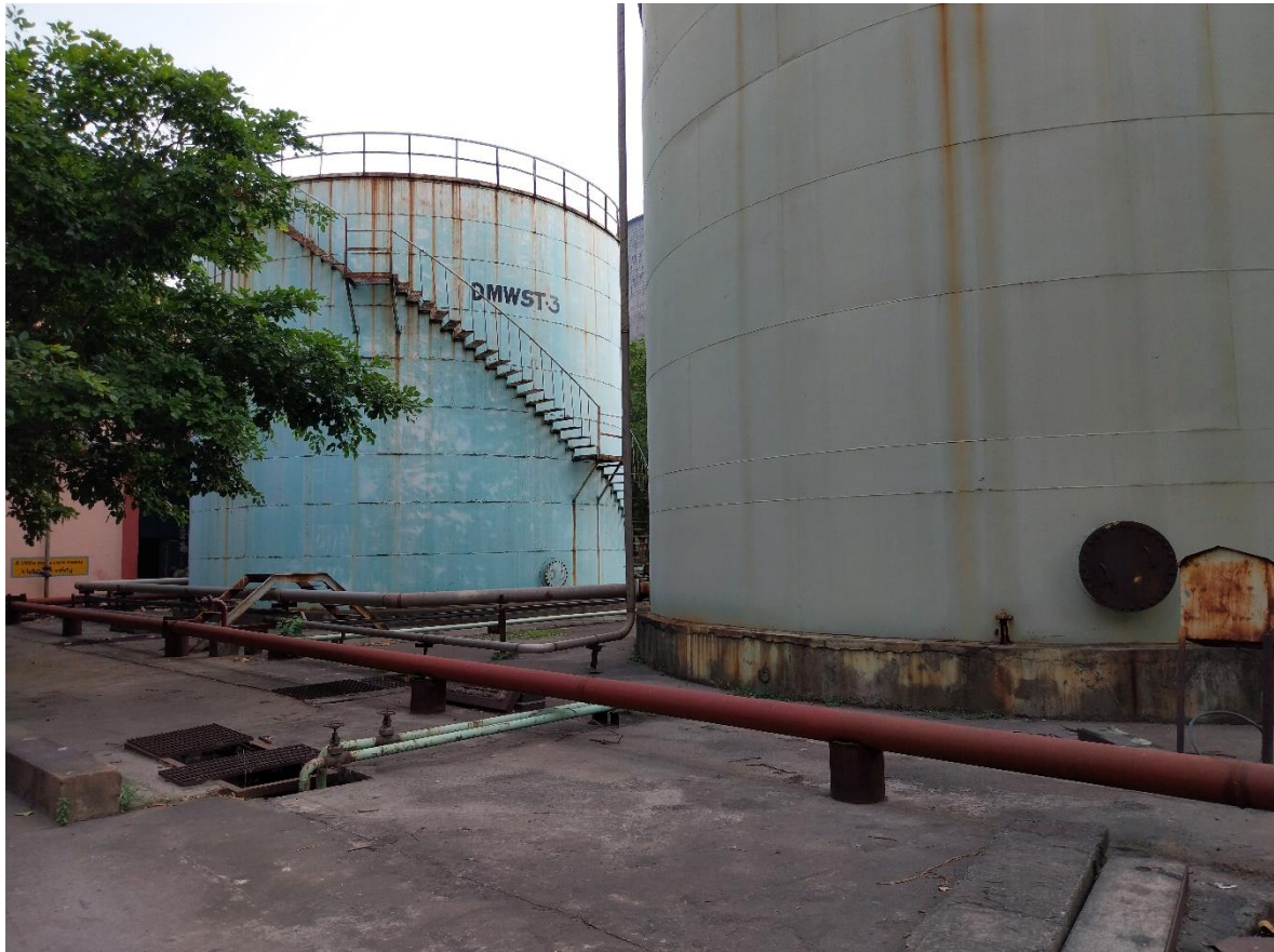
DM water treatment storage tank and transfer pump
