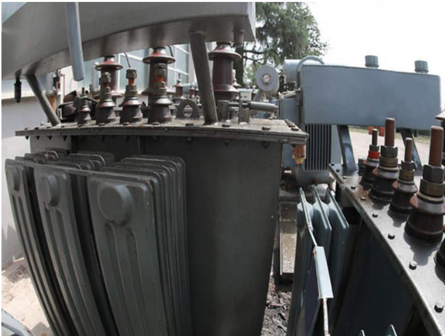
fig no.2.2 Transformer
