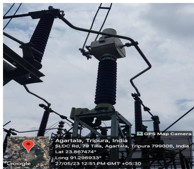
Fig: Current Transformer (CT)
