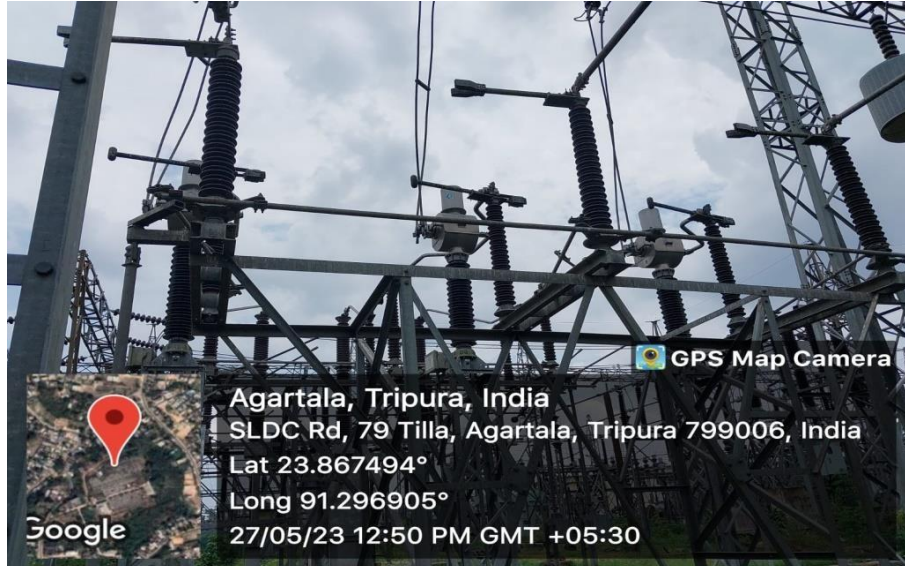
Fig: Capacitor Voltage Transformer
