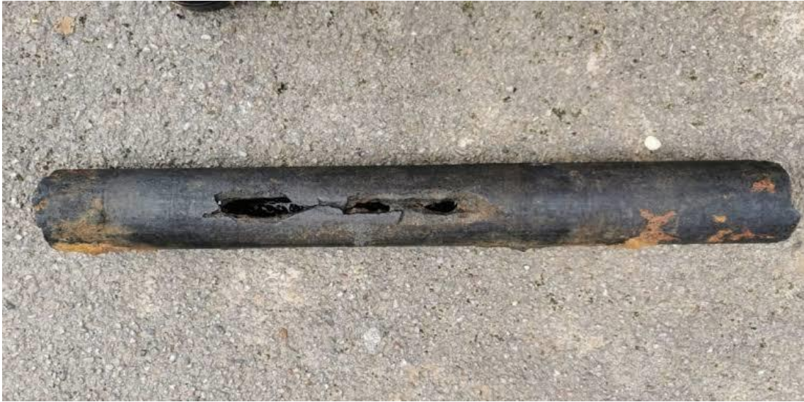
Fig 5.1 A Iron rod surface cracked Image
