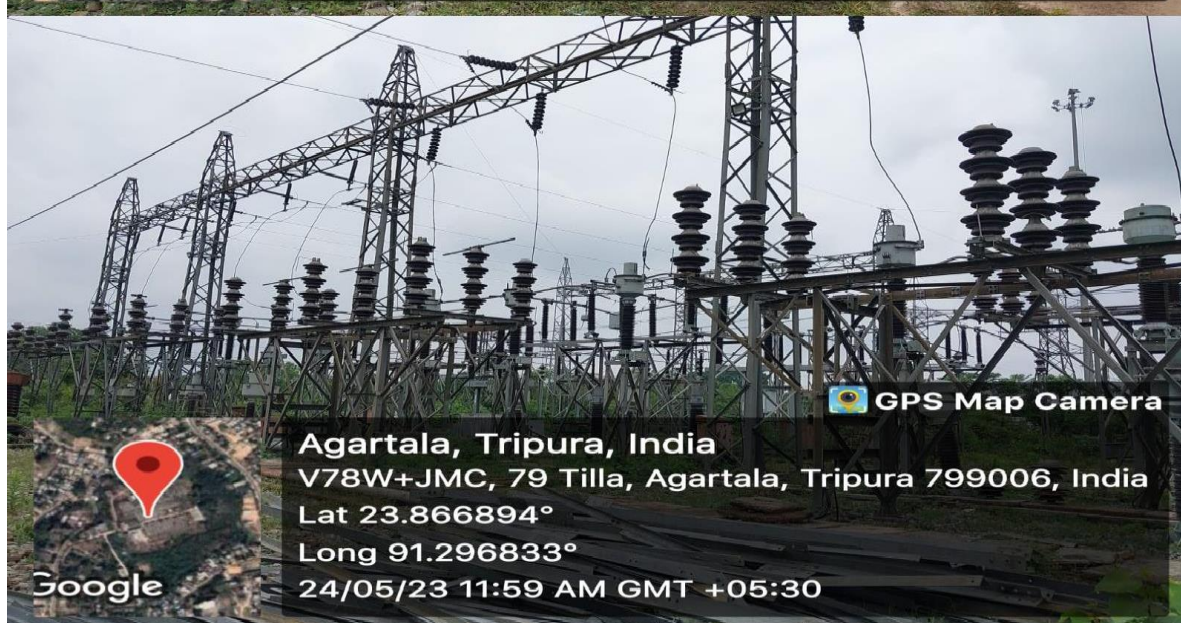
Fig: 132KV Grid Sub-Station Sub Division, 79 Tilla, Agartala, Tripura
