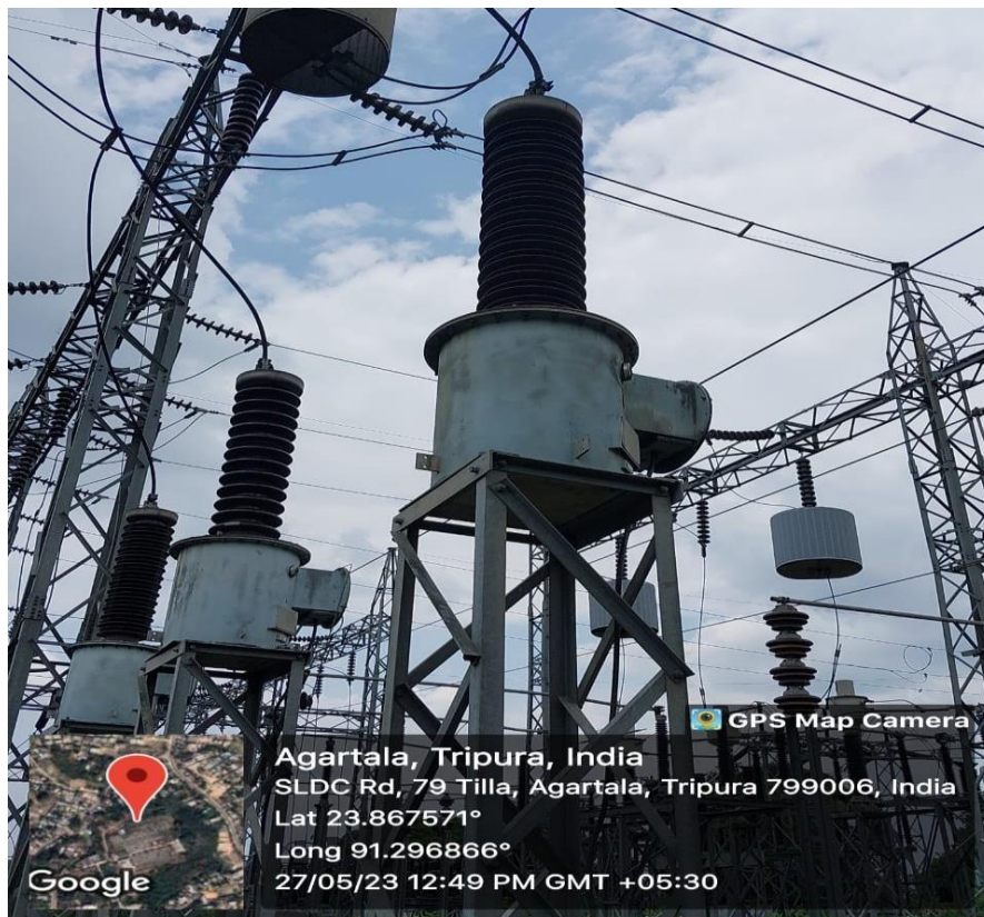
Fig- Potential Transformer (PT)
