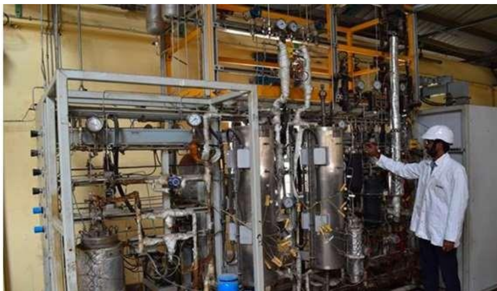
Figure 1 : Hydrocracking unit at CPCL
