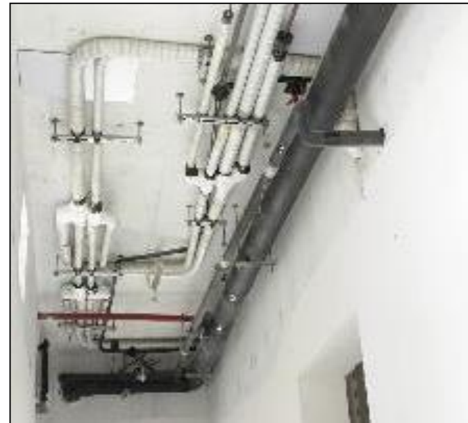
15 TH FLOR HVAC
