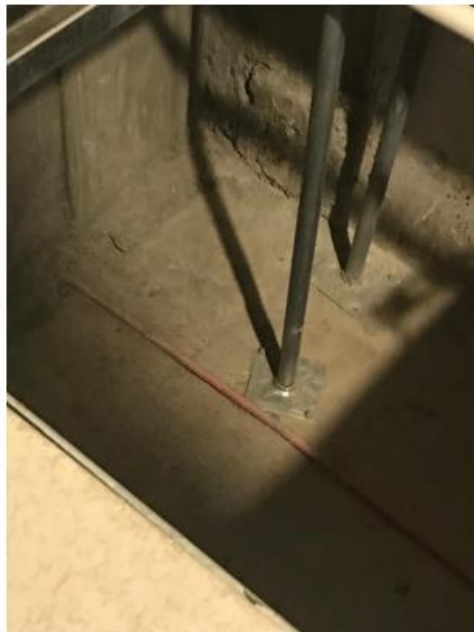
False flooring below whitewash
