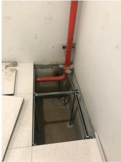
False flooring dampness
