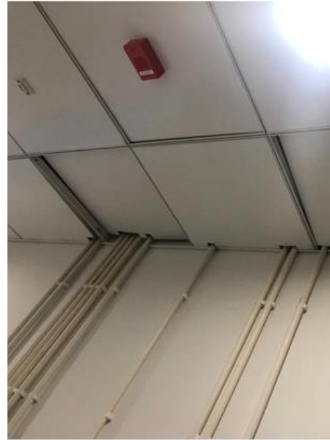
False ceiling alignment
