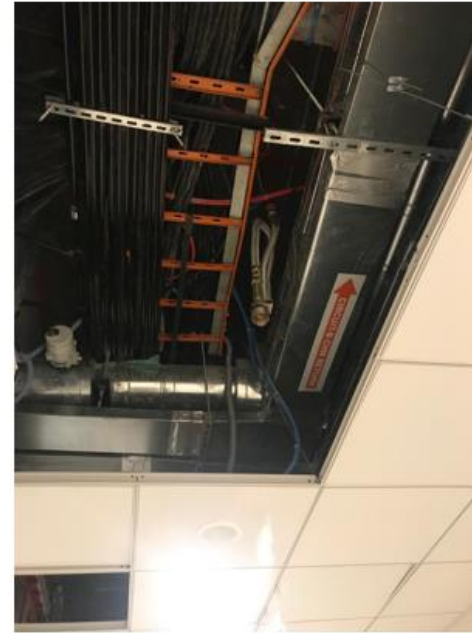
Ceiling support binding wire - GI wire to be provided
