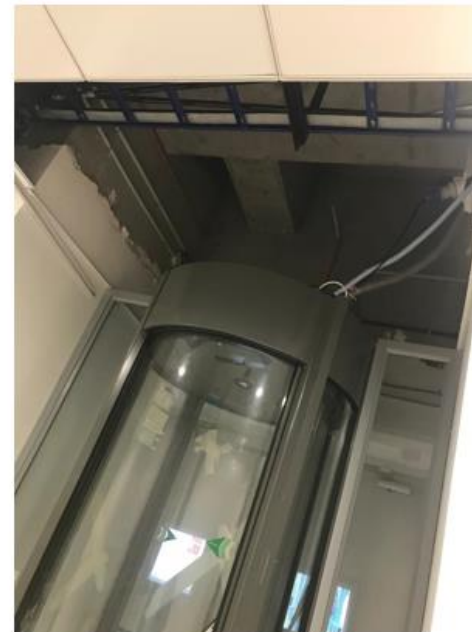
Mantrap above ceiling
