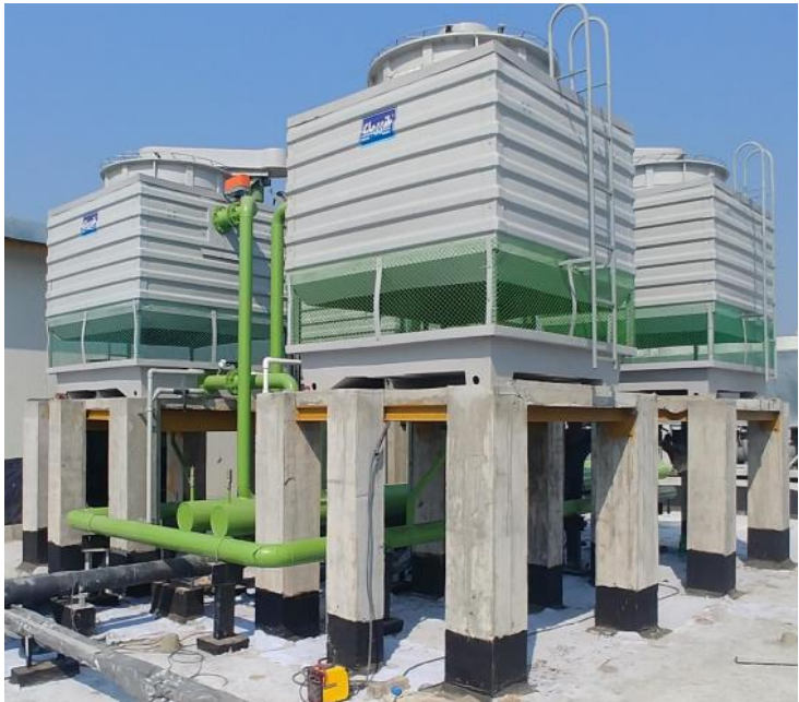
RESIDENTIAL BLOCK A - COOLING TOWER (WATER)
