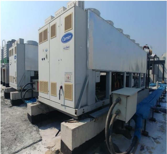
RESIDENTIAL BLOCK A - COOLING TOWER (AIR)
