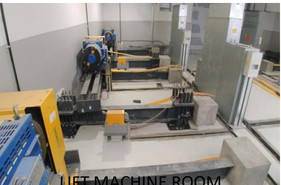
LIFT MACHINE ROOM
