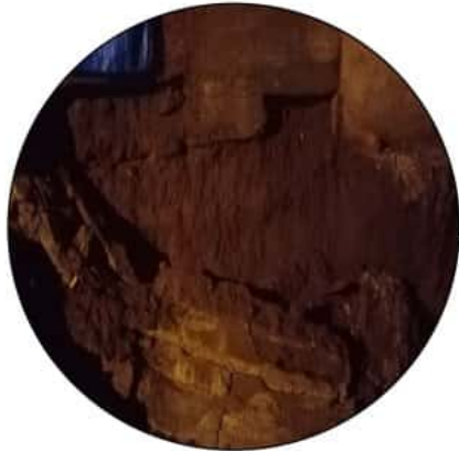
Movement of soil due to the rain caused landslide on construction site
