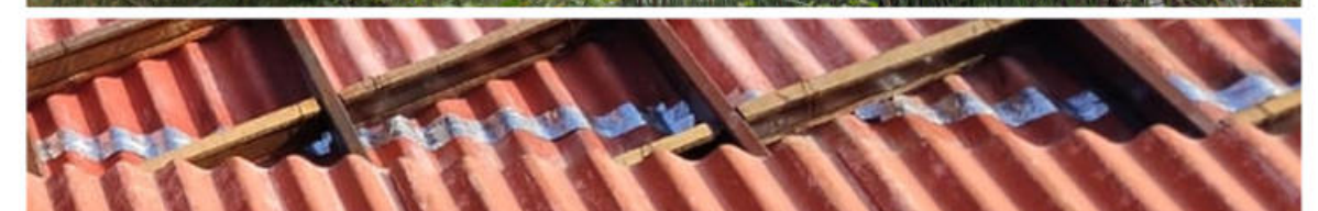
Tar sheet and metal tape sticking above asbestos sheet
