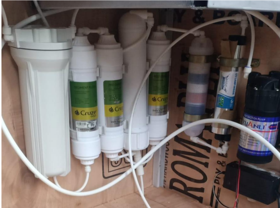
Figure 6.1 Whole Pipe Line and Membrane Connection Setup
