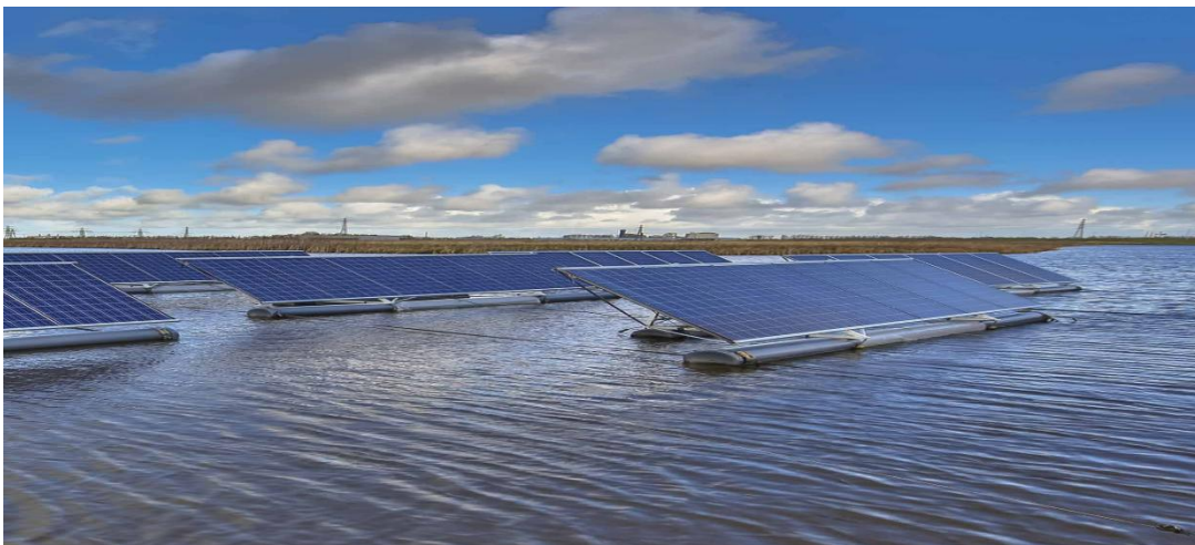
Fig 4.2: Solar Panels In Water Structure
