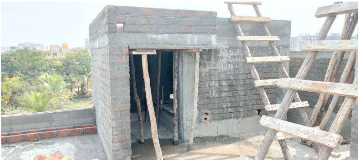
LIFT MOTOR ROOM
