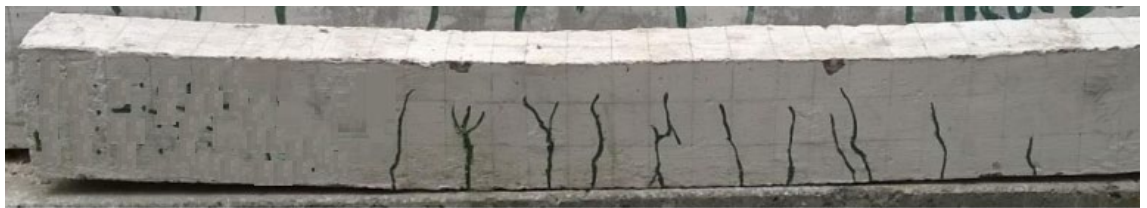
Fig 4.15 Crack pattern of NSCC
