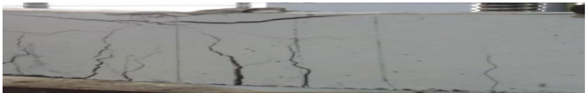
Fig 4.16 Crack pattern of RBASF1
