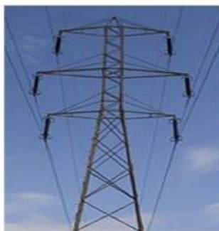
Power transmission line
