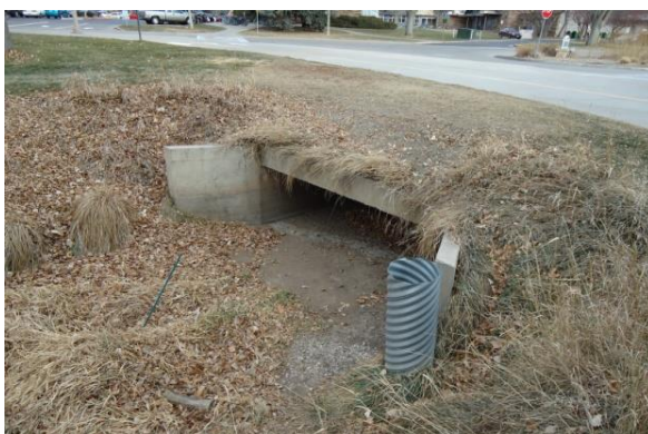
Figure 1.11 Poor maintenance blocking the culvert drain
